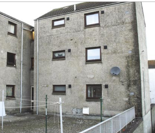
Forfar project with visible mould growth on wall
